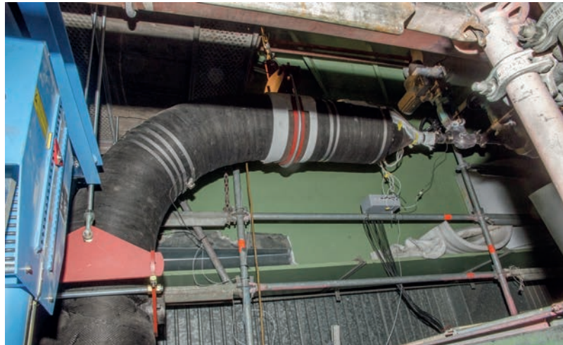
Fig. 8 Hybrid pipe elbow ( \varnothing \sim 320 mm) with an O-CMC ceramic fibre jacket ( t = 20 mm) with a total length \sim 4 m installed in a coal fired power plant
