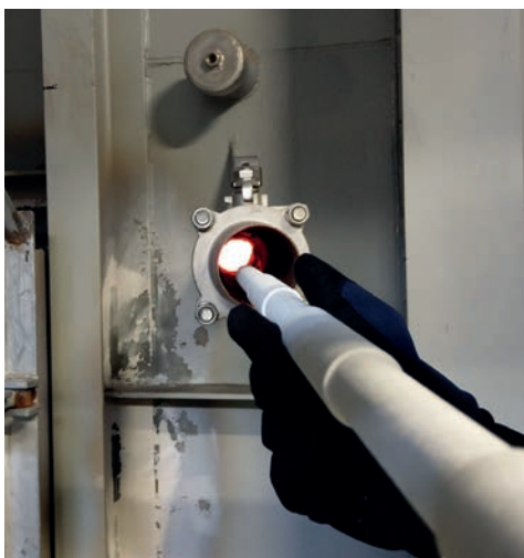
Fig. 11 Use of the ceramic lance for measuring the gas flow and gas composition in a waste incineration plant at MälarEnergi in Västerås/SE
